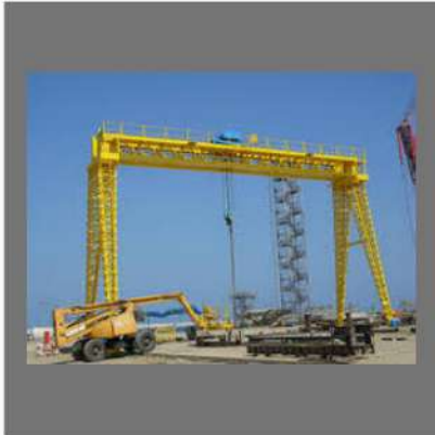
Gantry Crane (Heavy / Light)
