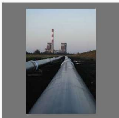
Pipe Line (air,oil,gas,water etc)
